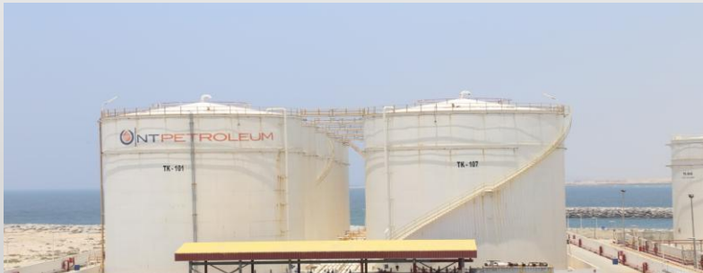
API 650 Steel Welded Storage Tanks
