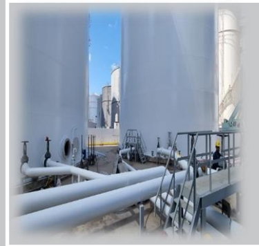
Above Ground Pipeline
